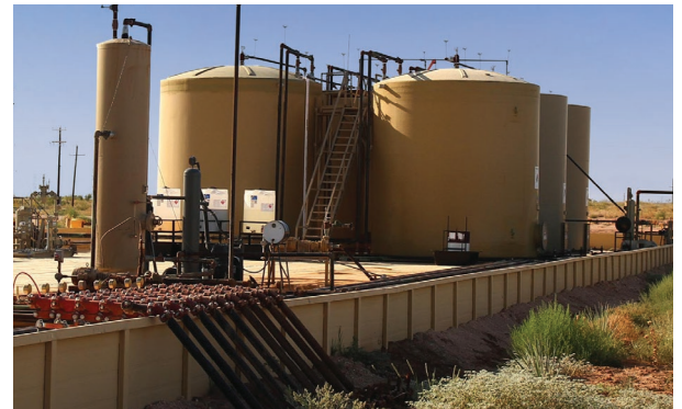
SITEGUARD secondary containment systems have been installed in more than 8,000 locations with a 100% environmental success rate.
